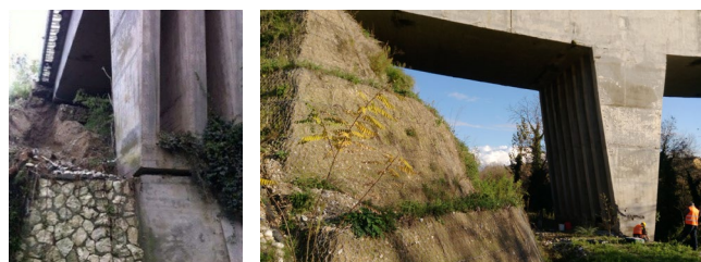
Figure 6. The landslide of the slope in 2015 and the armed lands behind the pier.
