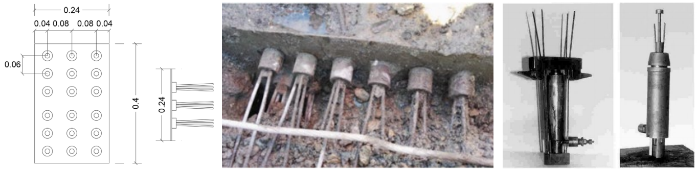
Figure 11. From the left: anchorage of two cables in groups of 3 wires, real picture in-situ , patent M1 and patent M4.
