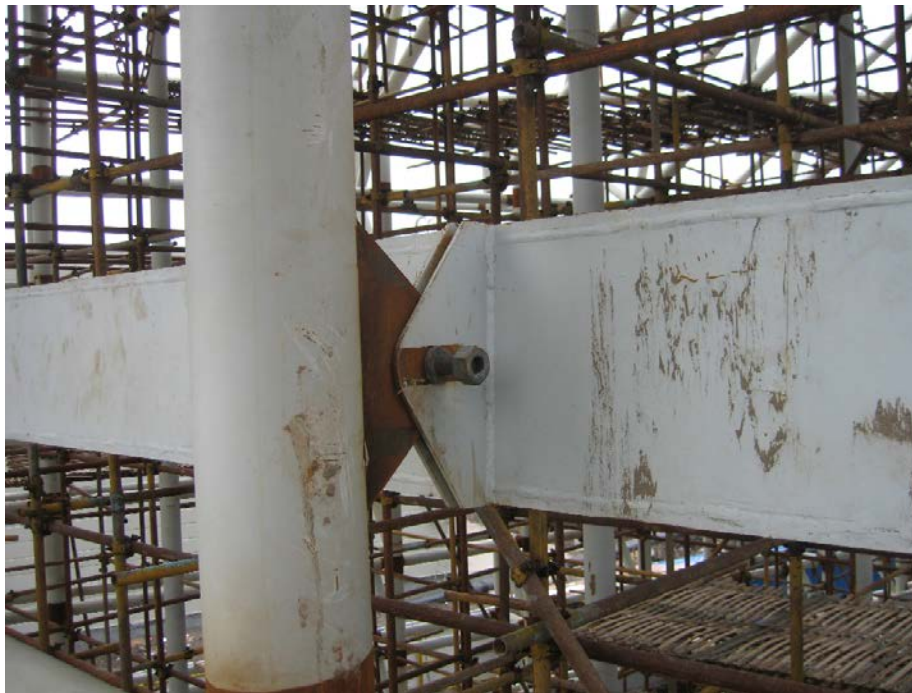
Figura 17. Unión bulonada en construcción, conectando viga de borde con tubo de fachada mediante orejetas Figure 17. Pin-bolt connection under construction, connecting the floor edge beam to the facade tube through ear-plates
