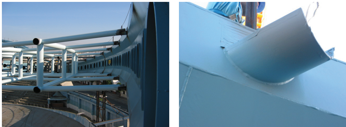
Figura 38. Unión de tubos a los cajones mediante teja metálica. Figure 38. Joint of the pipes to the caissons by means of metallic mesh.
