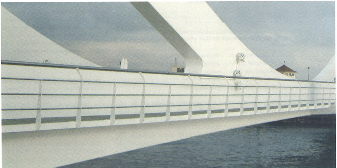
Fig. 6. Vista de la acera. Fig. 6. A view of the pedestrian foot walk.
